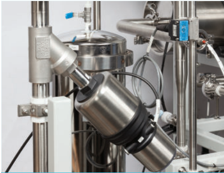
Automated self-adjusting modulating valves to control reject.
